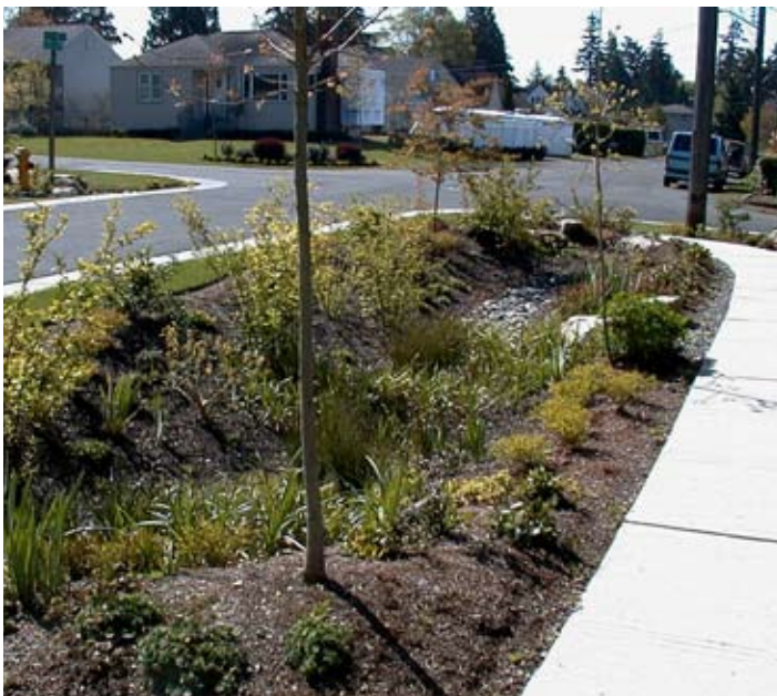
Street swales like this one above help to reduce the amount of stormwater runoff into the public sewer system.
