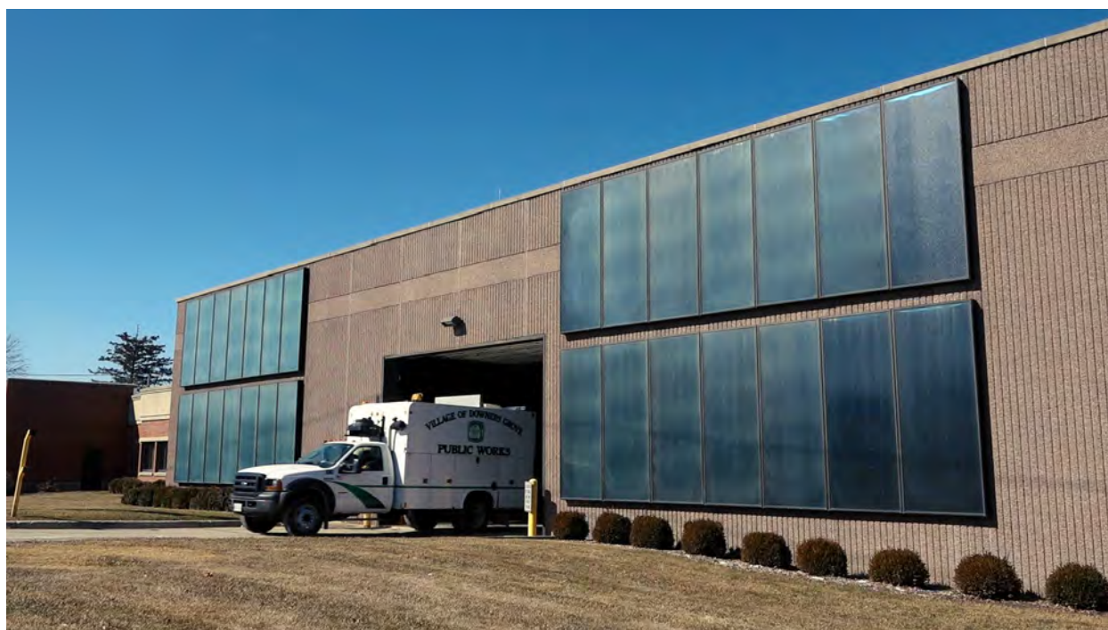
Solar panels on the Public Works building
