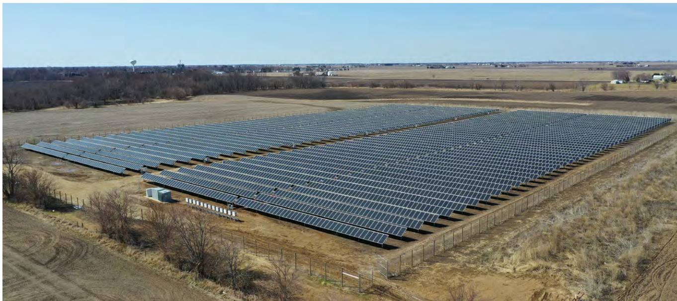
Figure 19. The 2.7MW Somonauk Road Community Solar project was developed in Somonauk by Nexamp, Inc. The project began producing clean energy to benefit subscribers in the ComEd territory in March of 2021. Image credit: Nexamp, Inc.
